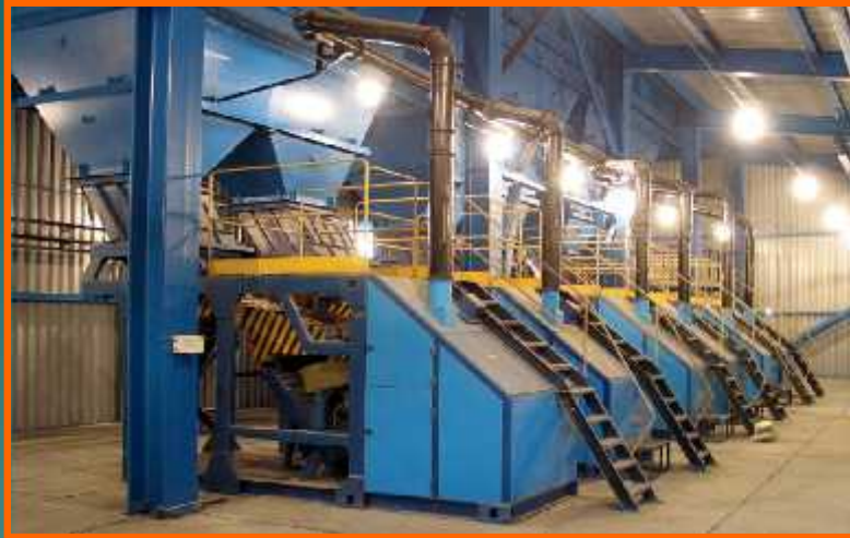
Separation Complex - Ural Mining and Metallurgical Company, Russia
